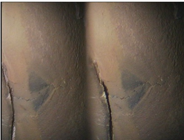
This photograph shows a crack in the trailing edge of a row two blade. This unit had 7658 Total Hours at the time of the inspection.
