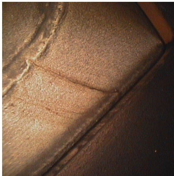
This view is showing a crack in a row two diaphragm ring segment.
